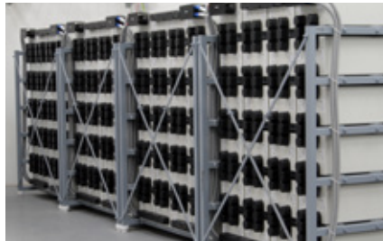
Energy Storage System
